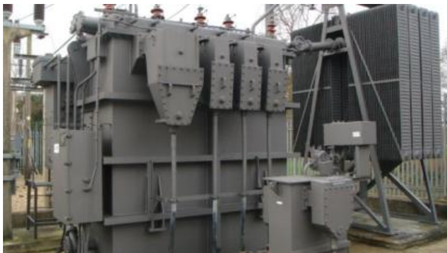
Photograph 2 – T2 33/11kV transformer at SSEPD's Purbrook primary substation
