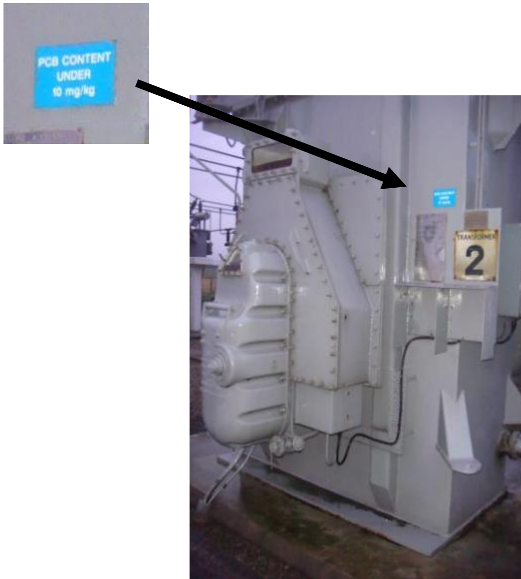
Photograph 4 – Example of PCB labelling on a 33/11kV transformer at SSEPD's Methlick primary substation
