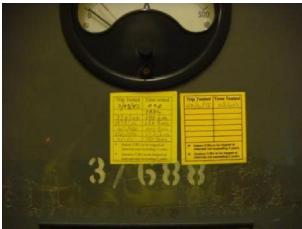
Photograph 6 – Example of trip-testing label at SSEPD's Lyndhurst primary substation
