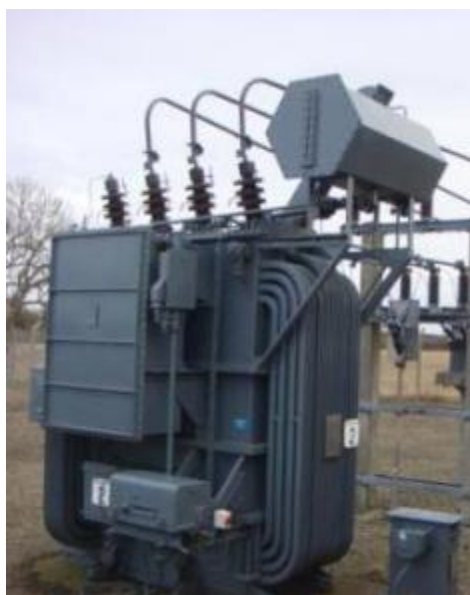
Photograph 1 – The 33/11kV transformer at SSEPD's Portsoy primary substation
