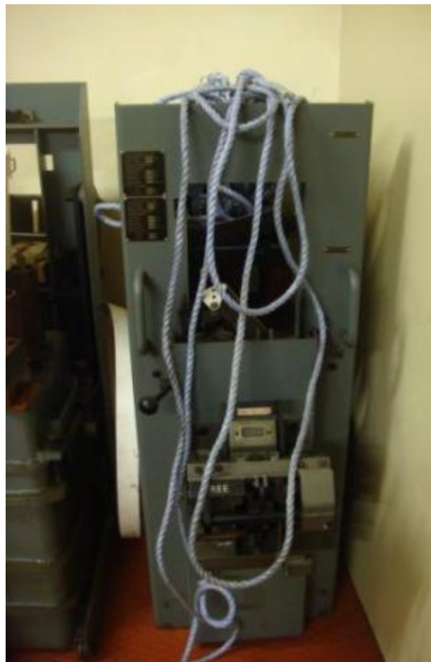
Photograph 8 – The rope used to close 11kV feeder circuit-breakers from outside the switchroom at SSEPD's Overgate primary substation
