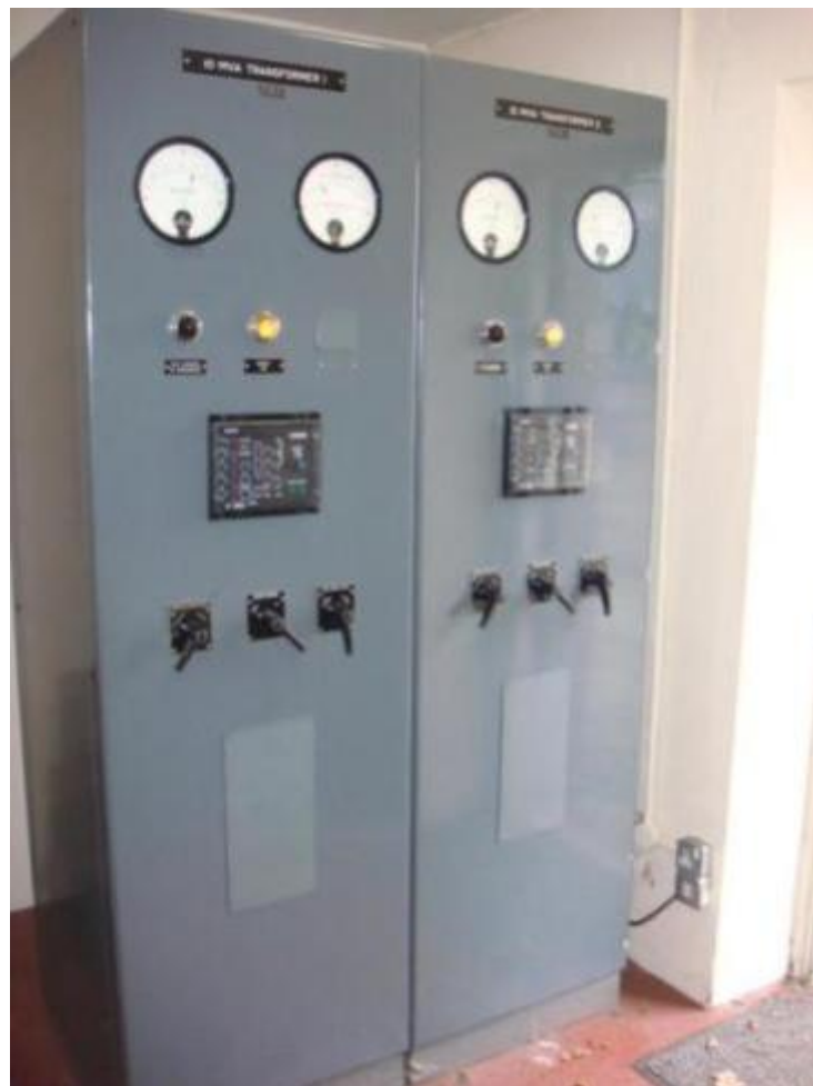
Photograph 5 – Example of modernised tap-change control equipment at SSEPD’s Craighton Cults primary substation
